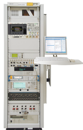
Figure 27. Automated test rack
